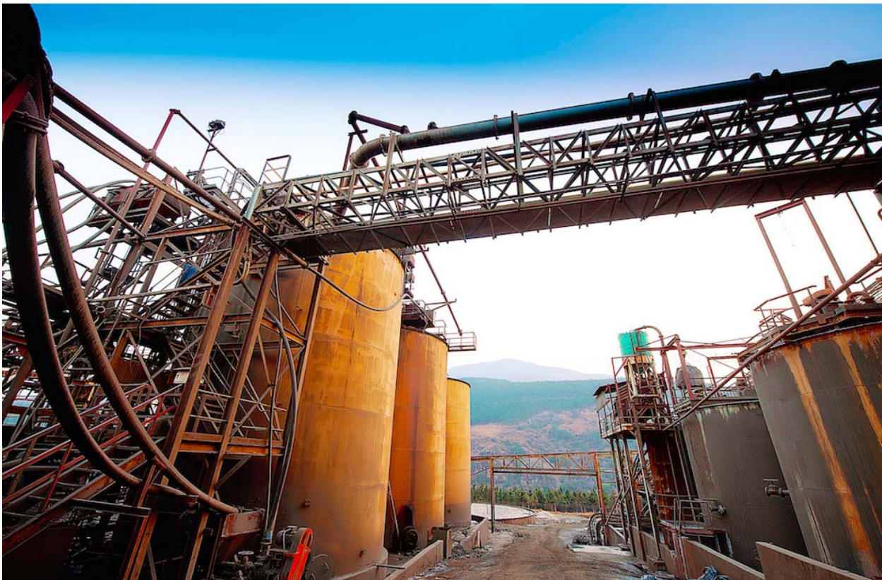
Figure1: Part of TGME plant picture
